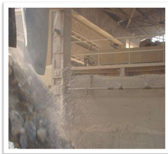
Water spraying System in Crusher Hopper
